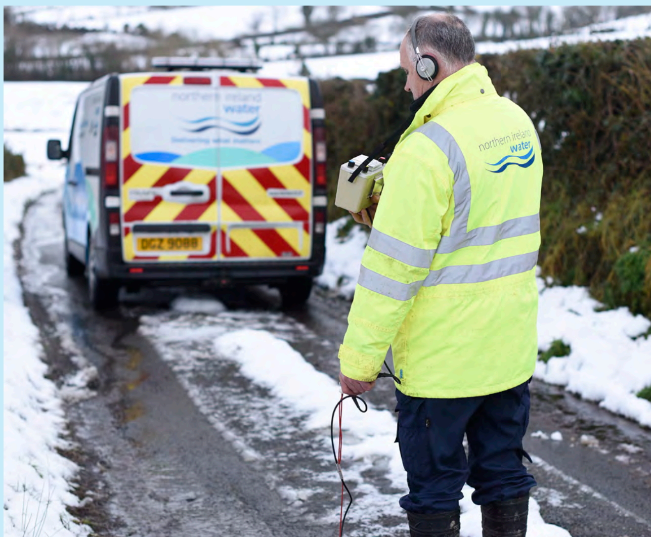
Leakage detection by NI Water staff member.
