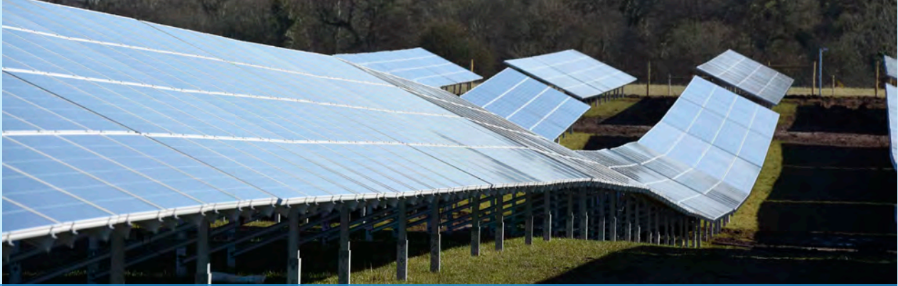
Solar panels at Dunore water treatment works, Co Antrim.
