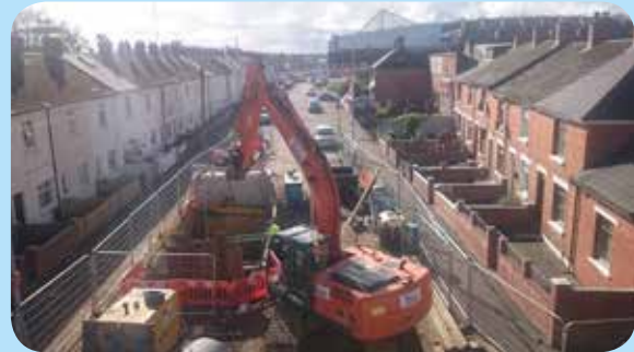
Aerial photo of the new storm sewer during construction at Donegal Avenue Belfast, Co. Antrim.
