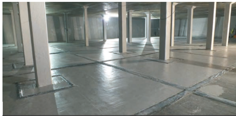
Interior of Ballyaghagan Service Reservoir, Belfast.
