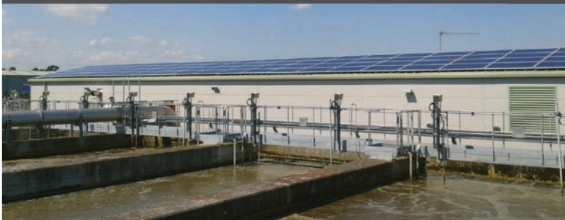
84 solar panels installed on the roof of Antrim Wastewater Treatment Works, Co Antrim.
