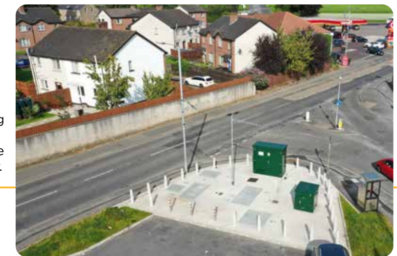
New wastewater pumping station in the west of Armagh City, County Armagh
