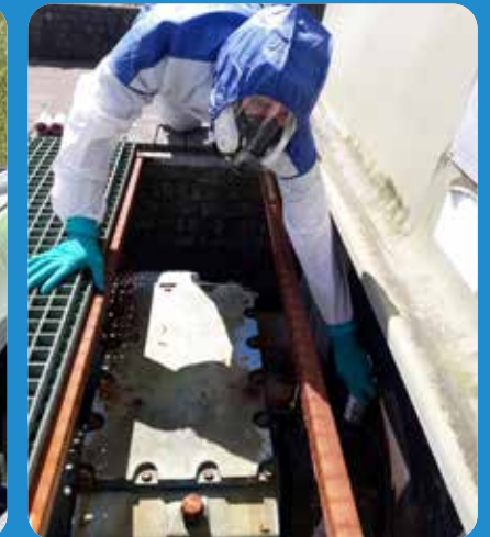
Mechanical and electrical operative fitting a greaser
