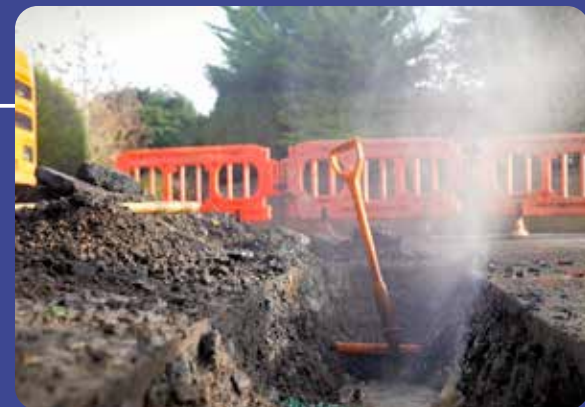
Water leaking from a burst pipe
