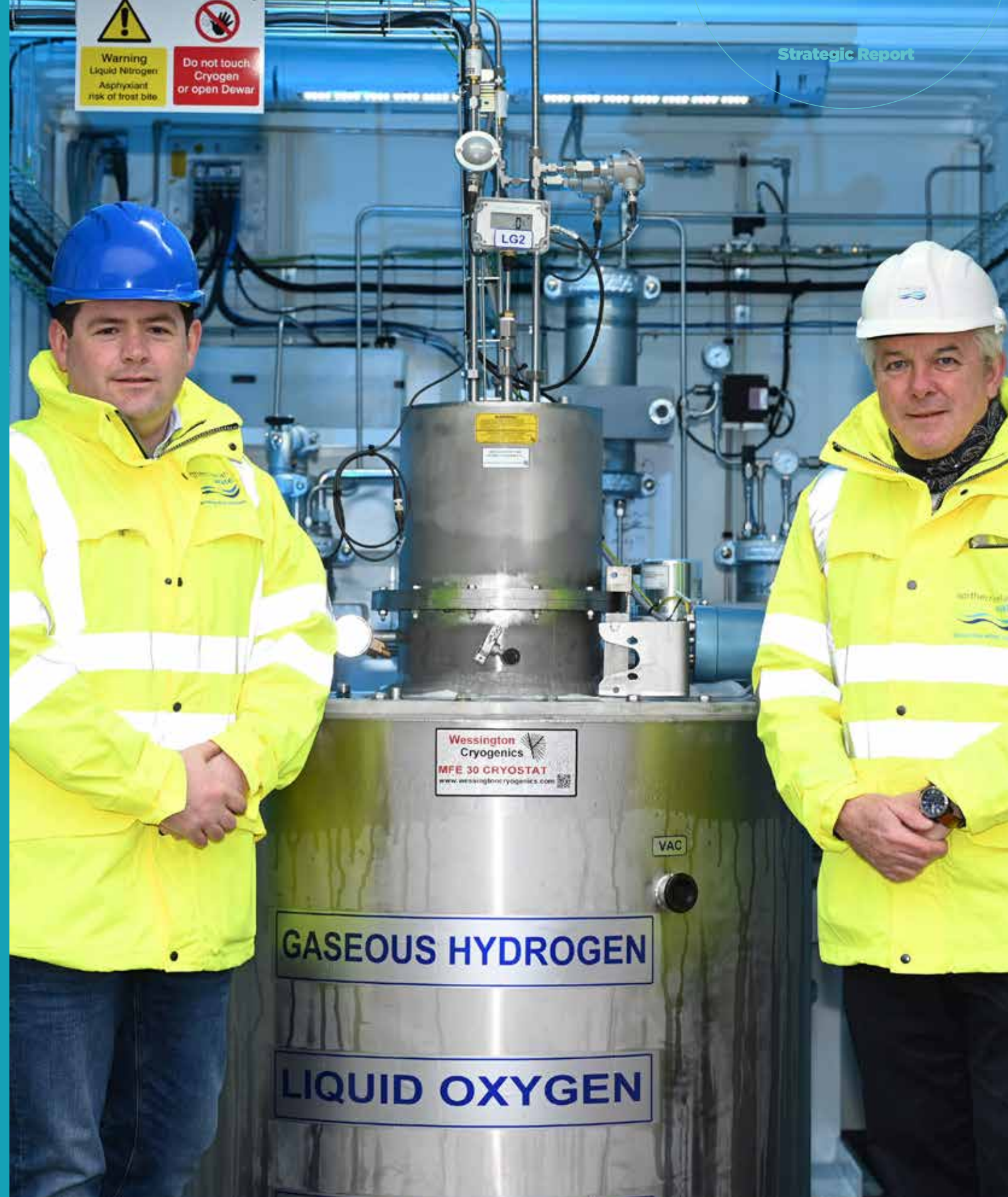
Electrolyser at Kinnegar wastewater treatment works, Holywood, County Down
