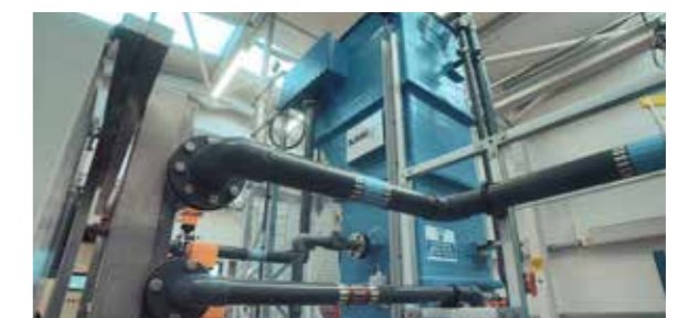
New treatment plant at Rathlin Island, off the coast of County Antrim
