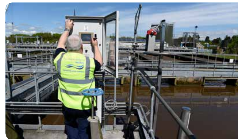
Real time control technology at Antrim used water treatment works, County Antrim
