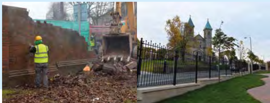
COVER IMAGE and RIGHT : Before and after pictures of a long standing Peace Wall on the Crumlin Road in North Belfast, which was removed in 2016.
