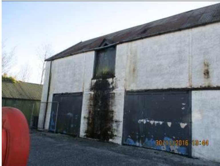
Photograph 8 View of shed openings with clear signs of continuous water damage from the first floor opening.
