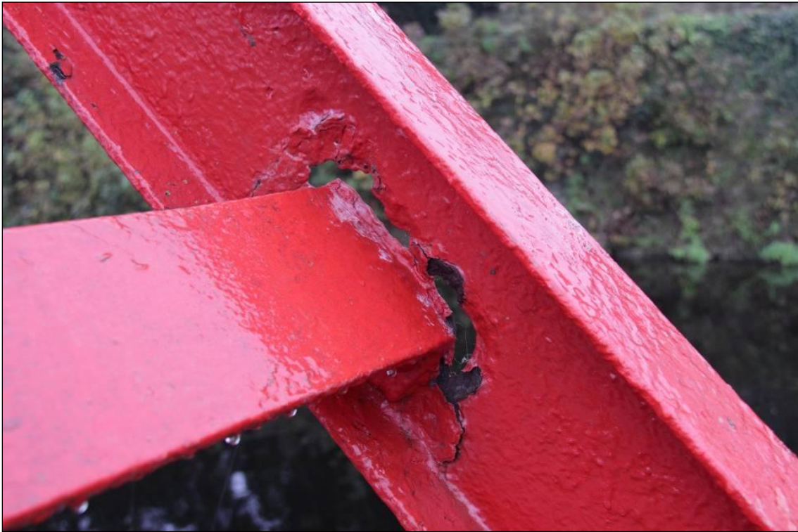
Photo 7 - Necessary Structural Repairs to Ironwork
