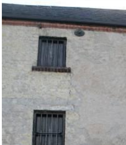
Photograph 3 Vertical crack between 1 st and 2 nd floors
