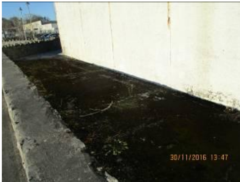
Photograph 3 View of ground level around perimeter of shed, concrete finish with no drainage channels
