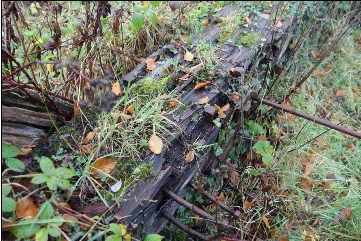
Photo 4 - Main Sliding Timber - Severe Rot
