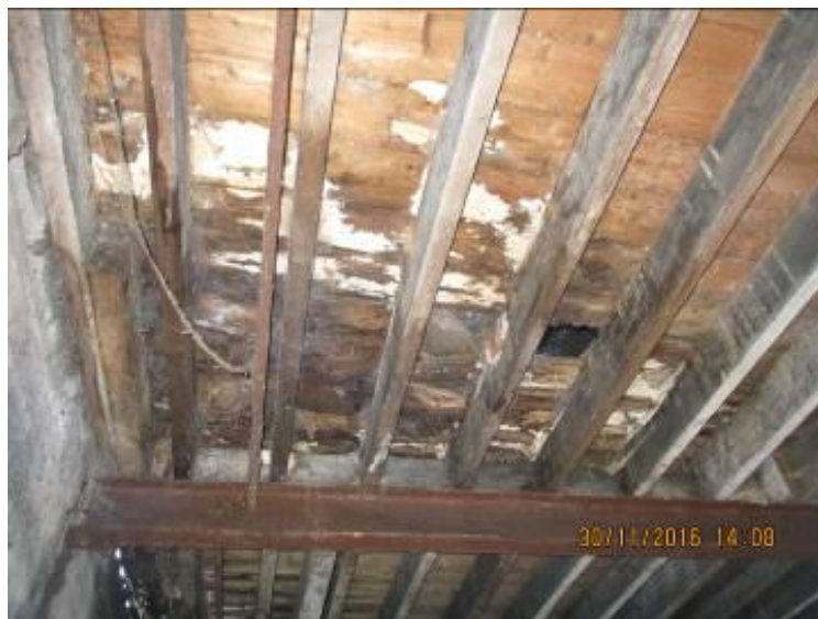
Photograph 2 View of wet rot to first floor timber floorboards.
