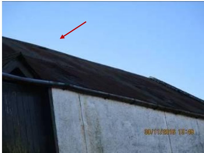
Photograph 1 View of rear roof plane with loose roll top ridge highlighted
