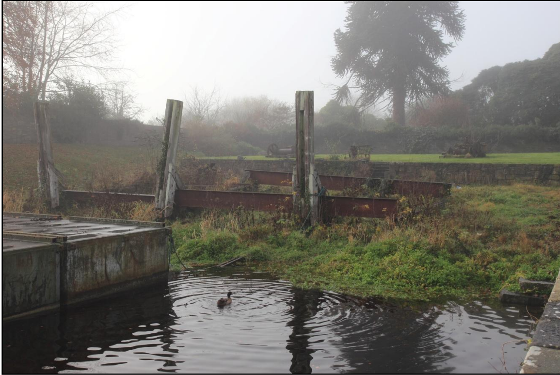
Photo 8 - Upright Sections in Poor Condition
