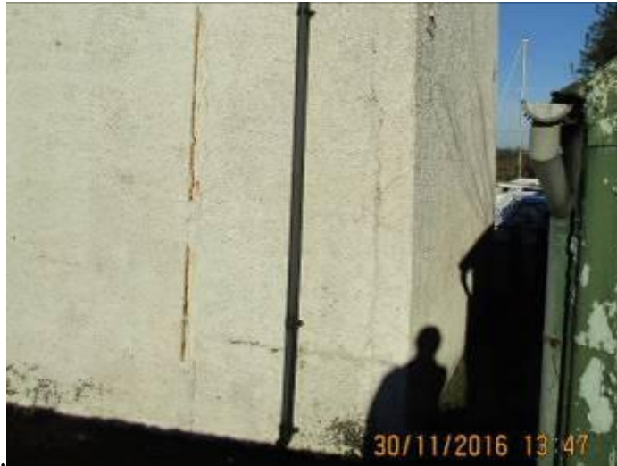
Photograph 6 View of render to front of building with cracking and crazing on view
