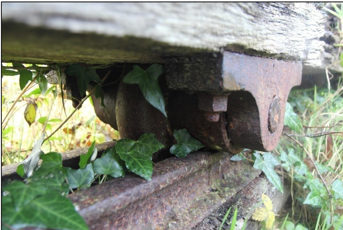
Photo 7 - Main Beam Wheel/Runner
