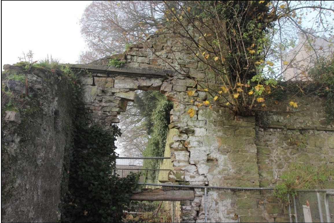
Photo 2 - Damaged Corner of Cathedral Wall
