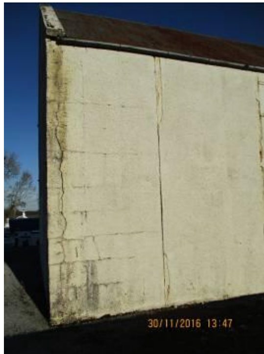
Photograph 7 View of patent crack defect.
