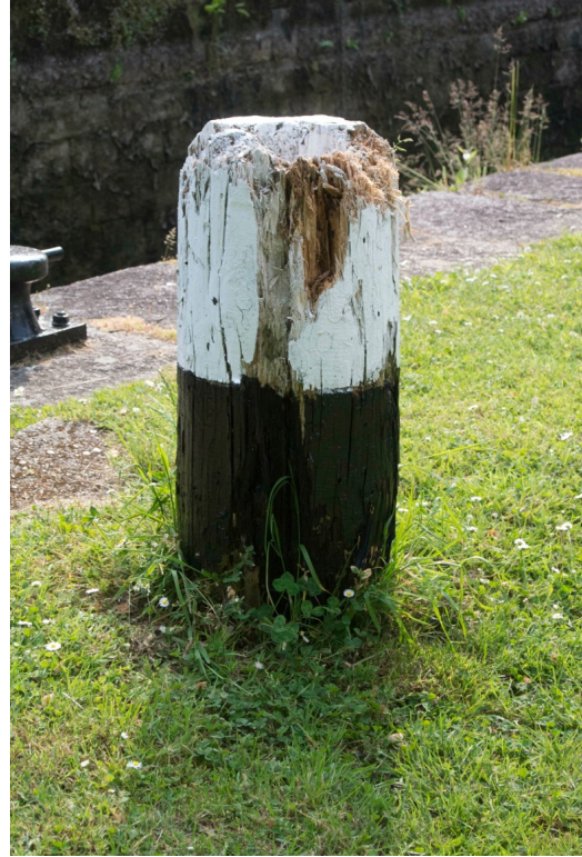
A replacement softwood post, now severely decayed. A protective membrane would prolong the life of the timber
