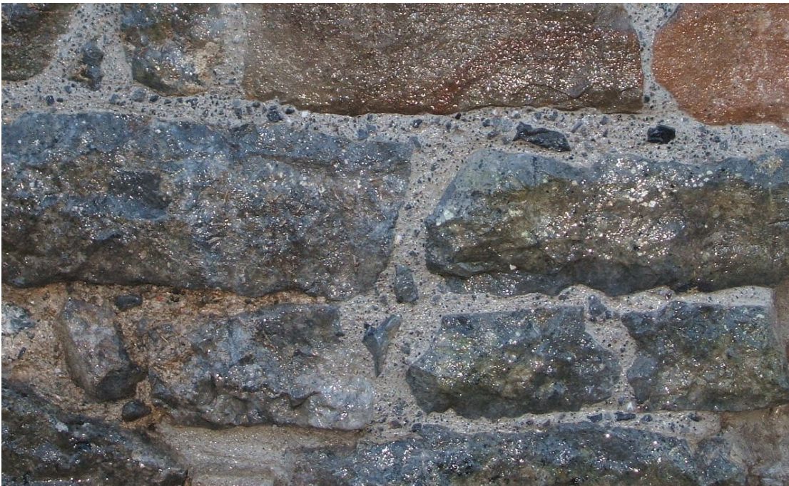
A good example of new pointing repair with pinnings. Joint beaten back to compact mortar, expose aggregate and stone edges. Note the good match with the older pointing on bottom left
