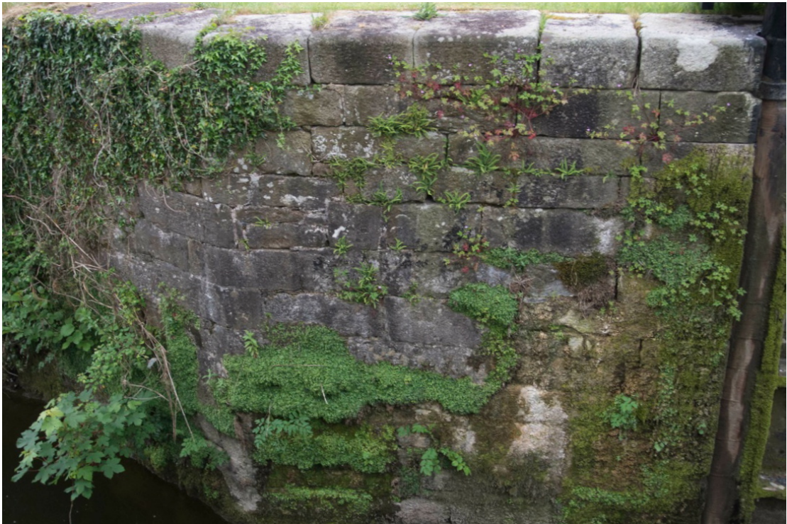
A canal lock wing wall showing the full range of vegetation - aquatic plants, moss, ivy and self-seeded sycamores. Note the number of joints that are empty of mortar
