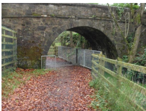
Figure 4: a simple railing pushes users out from the low side of the arch. Railings and fencing prevent any watery mishaps!
