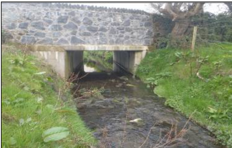
Photo 5.3.1.2 - Rivers Agency upgraded accommodation bridge on the Halfpenny River downstream of the Knockramer Meadows Development.
