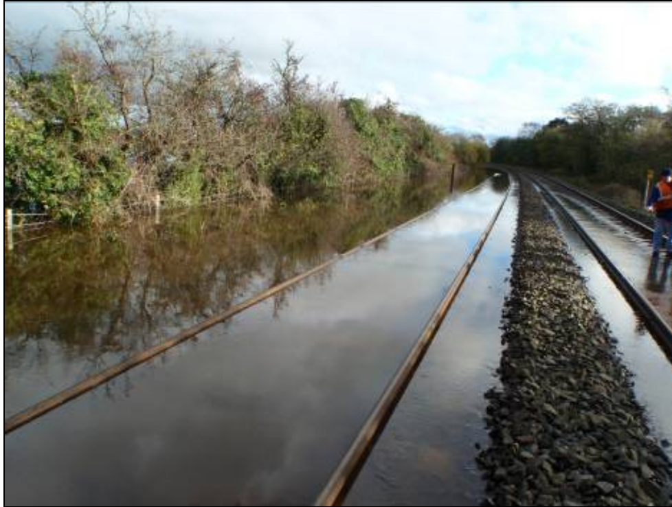
Photo 5.8.2.1 - Portadown railway line flooded in Oct 2011
