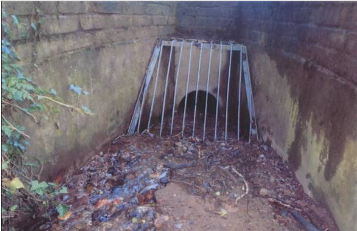
Photograph 5.5.6.1 - Ongoing problem with gravel accumulation at Ferndene Stream
