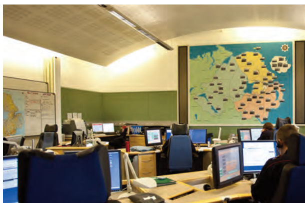
Regional Control Centre
