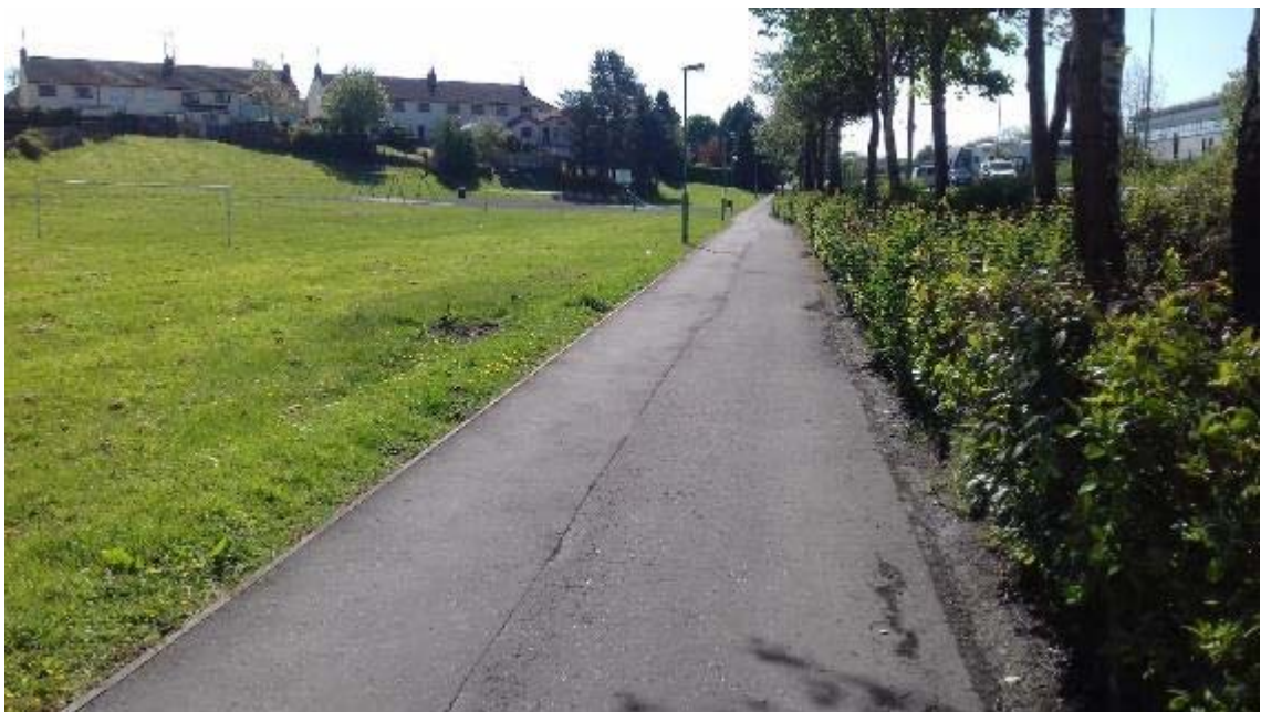
Photograph 31: Offline Footway adjacent to the A5 Great Northern Link (See Drawing D-021)
