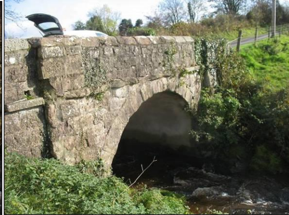
Photograph 3.3.5-2 - Routing Burn Downstream of the Existing bridge (approx. 265 m downstream of Proposed Scheme Crossing)
