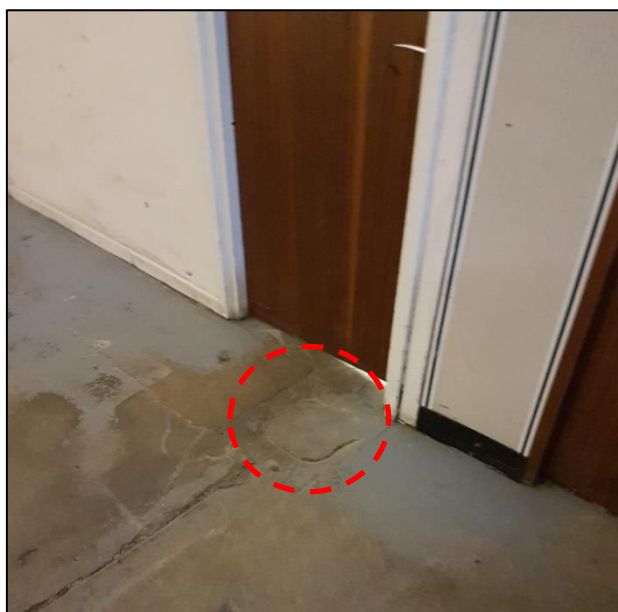
Picture 6.1 Redundant sealed floor gully inside Print Press building
