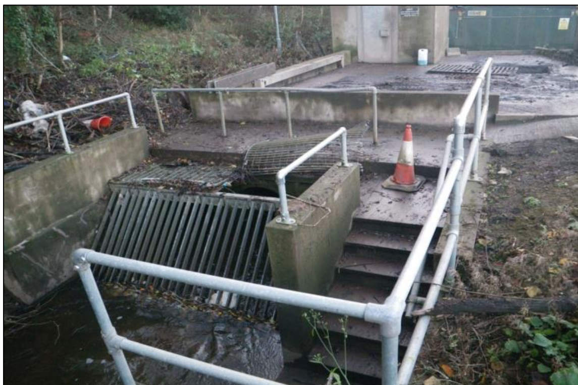
Picture 6.2 Inlet to culvert showing platform removed (DfI Rivers Flooding Incident Report)
