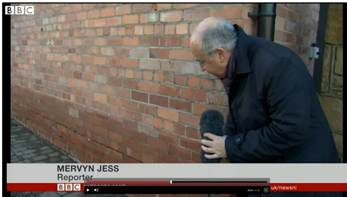
Picture 6.4 Screenshot from BBC News footage showing depth of flooding at east end of “The Weaving Sheds” building (BBC)
