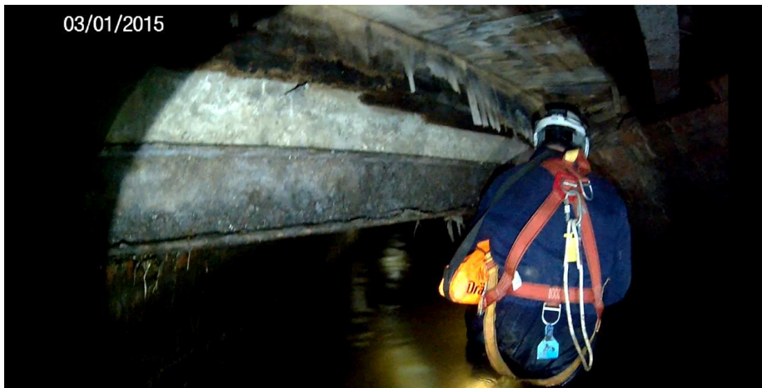
Picture 9.1 Obstruction across culvert upstream of manhole U4304/05
