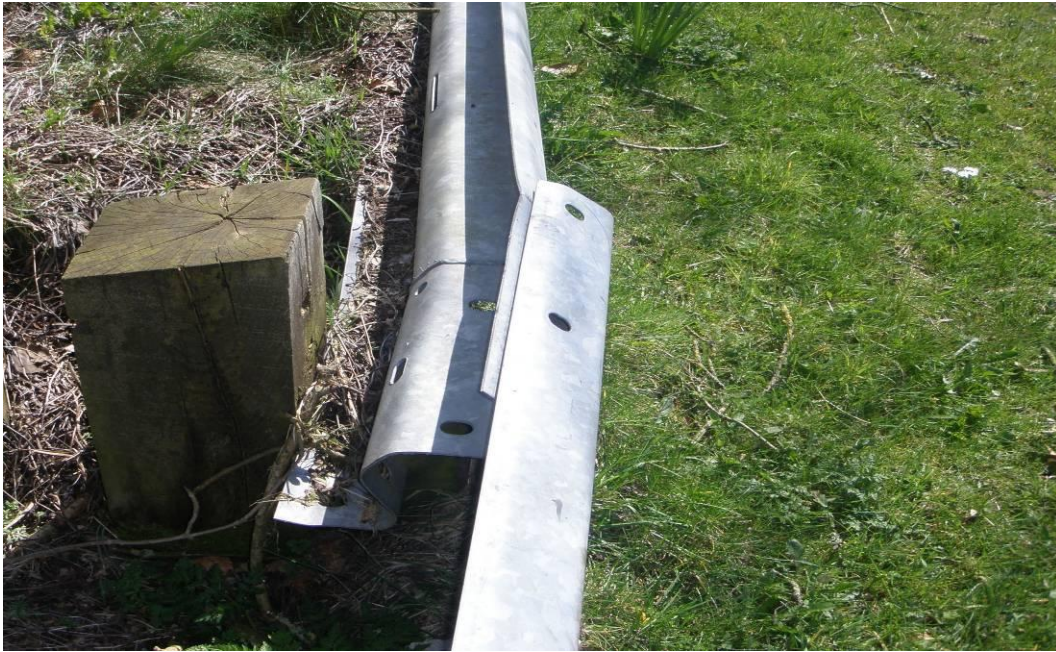
Wooden post, blocked out piece missing, barrier not connected to post, top of rail low, all bolts/fixings missing.
