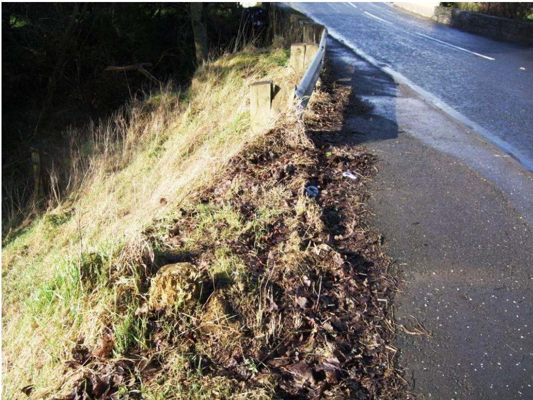
No Approach Terminal, Rotten Wooden Posts, Hazard within working width, insufficient length of hazard protection.
