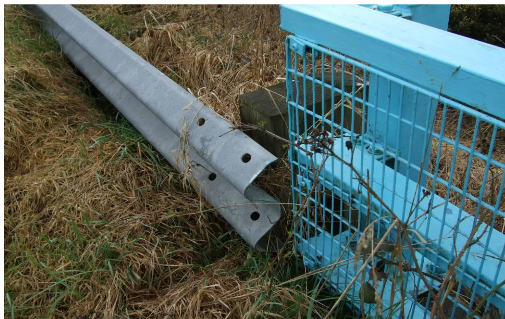
Beam is not attached to post No connection to parapet Barrier and parapet misaligned
