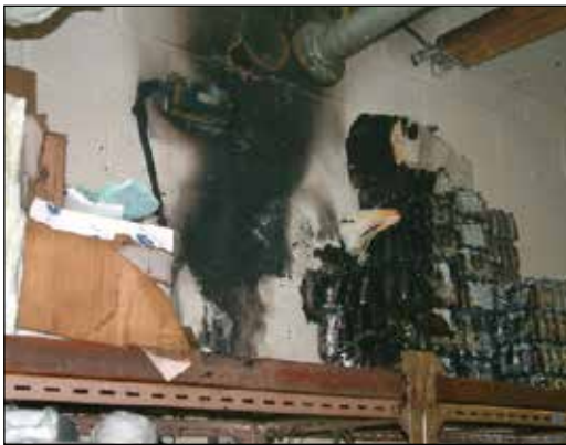
Figure 4: Fire in a storeroom (hot works)
