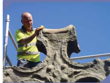
Conservation work at Donaghmore to prevent water egress at top of the cross, Photo: NIEA
