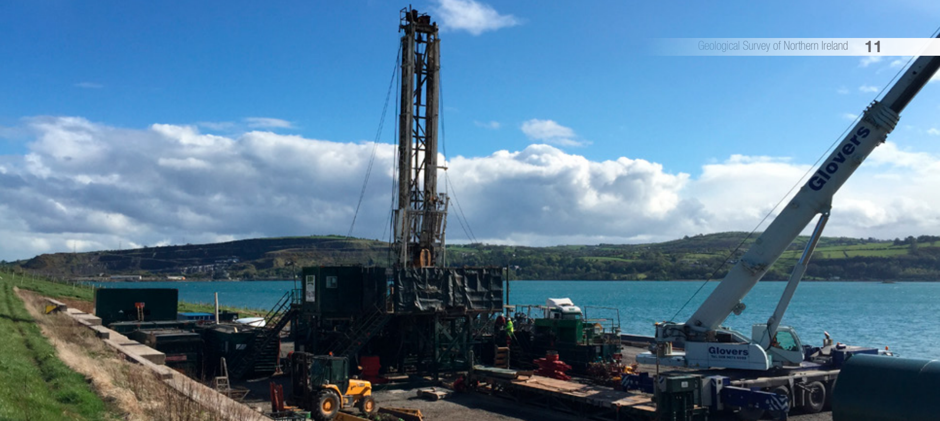
Islandmagee well site. Courtesy of Islandmage Storage Limited.
