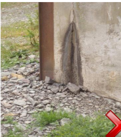
Photo 6 - Leaking silage clamp
