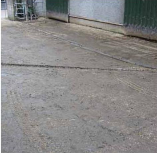
Photo 25 – Run-off from a frequently used collecting yard is slurry.
