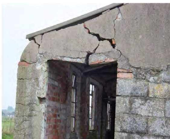
Figure 28. Damage to a doorway at the squadron armoury, Mullaghmore, Co. Londonderry (DHR 00075:041)
