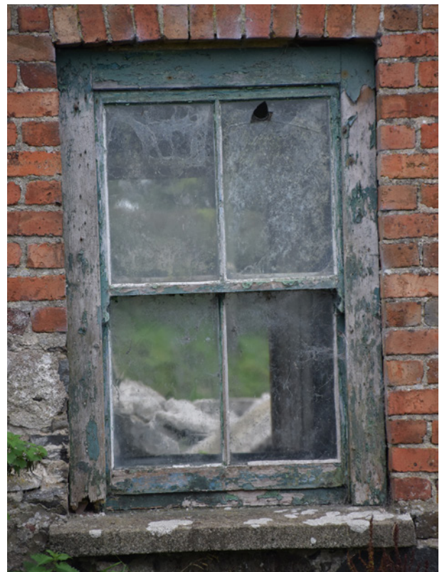
Window not properly maintained and beginning to rot.
