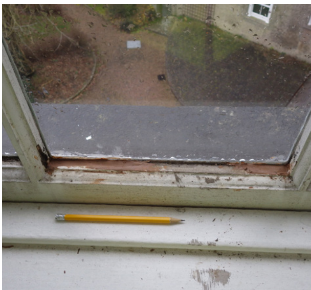
Horizontal areas are often most vulnerable.
