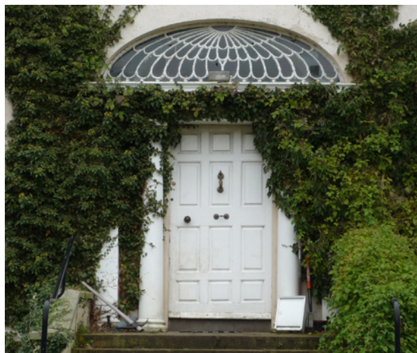
Detailed Fanlights require a specialist to repair.
