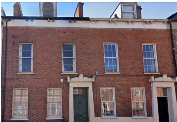
Replacement PVC-u windows (sash and dormer on the right) can alter the appearance of a terrace.
