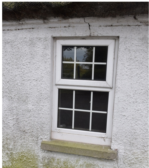
Inappropriate PVC-u replacement window detracting from the character of the building.
