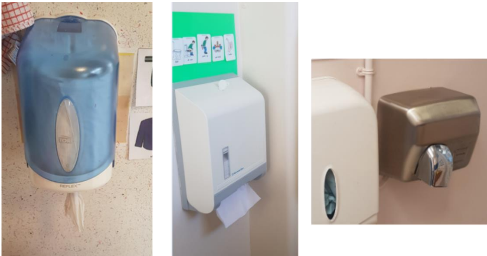
Figure 12. Examples of wall-mounted paper towel dispensers and hand dryers in different preschools.
