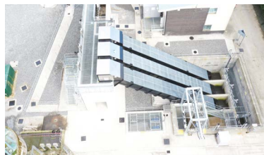
Strabane Wastewater Treatment Works, which has seen an upgrade of the existing treatment facility to include: installation of a new inlet works, pumping station and fine screening equipment to protect the water environment.
