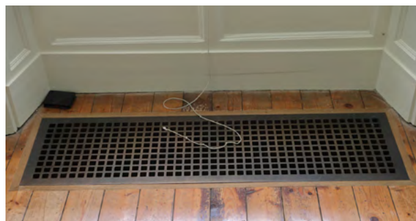
Vent in floor, heat source unknown
