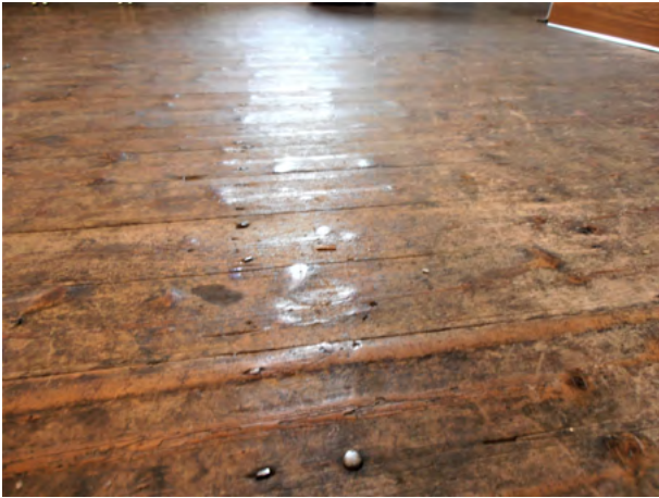
Worn floor boards
