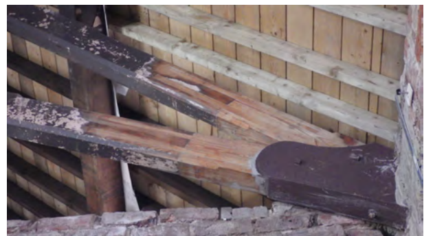
Image shows principle of repair to structure, this repair to truss footings
