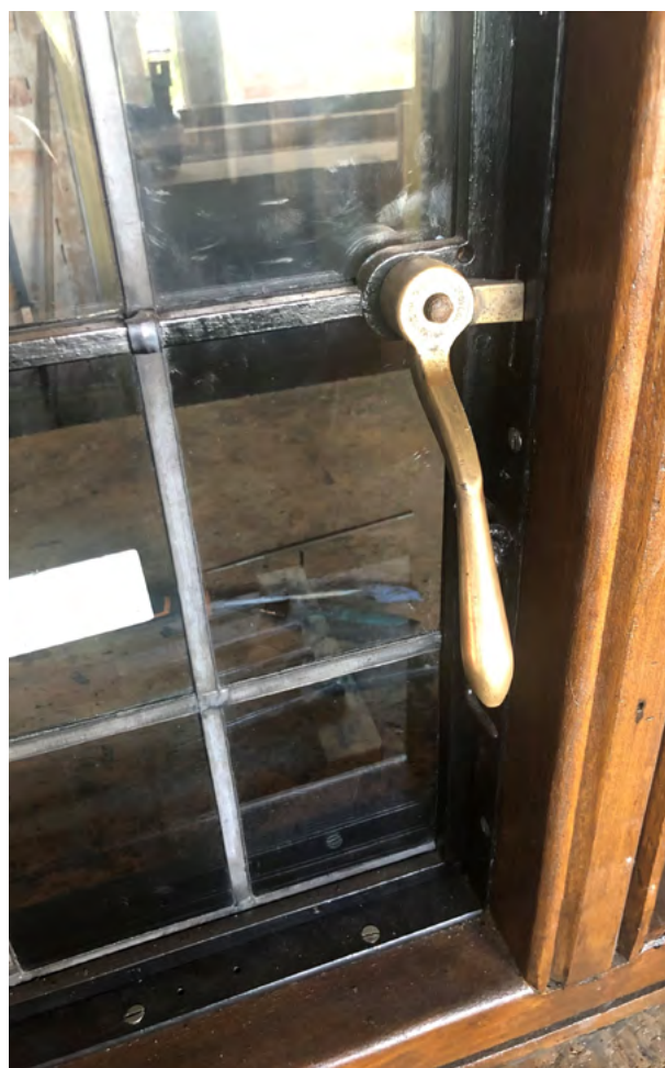
Protruding historic stay
