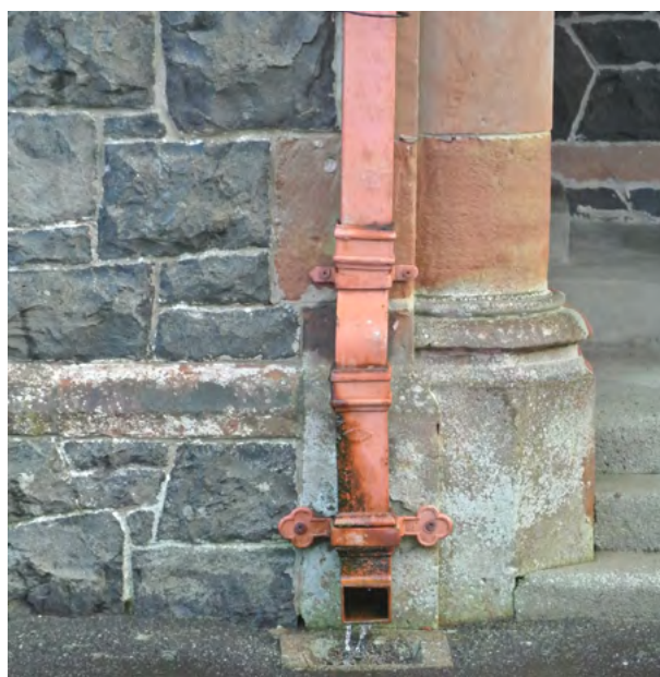
Cast iron downpipe discharging into gully and keeping the base of the wall dry
