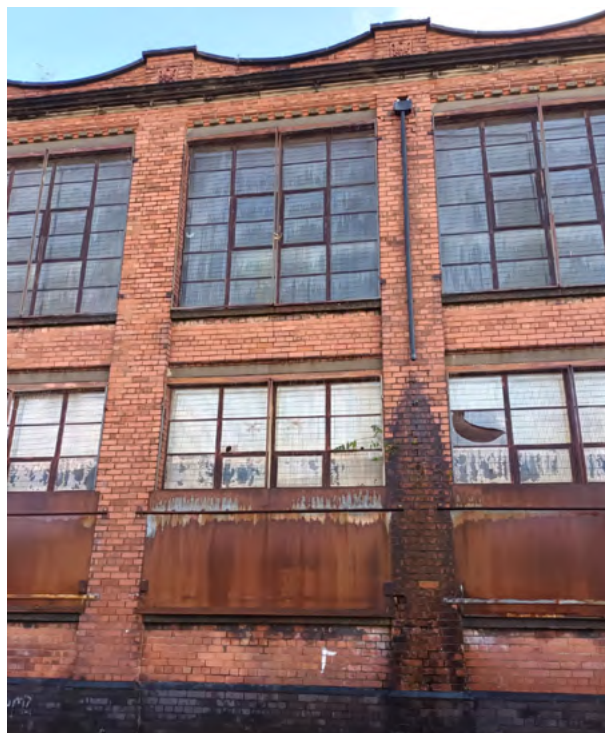
Missing downpipe which has caused damage and staining to the brickwork, and wall saturation
