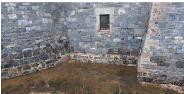
Extreme case of water not draining from building perimeter; in this case due to a broken culvert, water is able to soak into the wall
