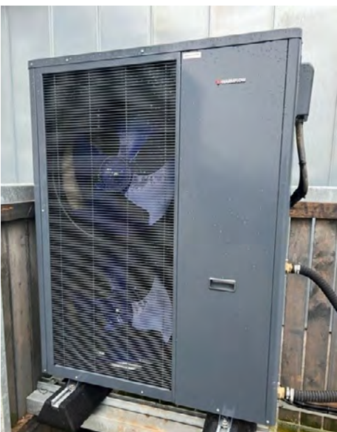
Heat pump at Caledon Wool Store
