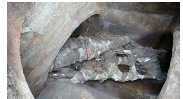
Figure 8 - Set of ladders discovered in a sewer and covered in sewage related debris in Derry/Londonderry
