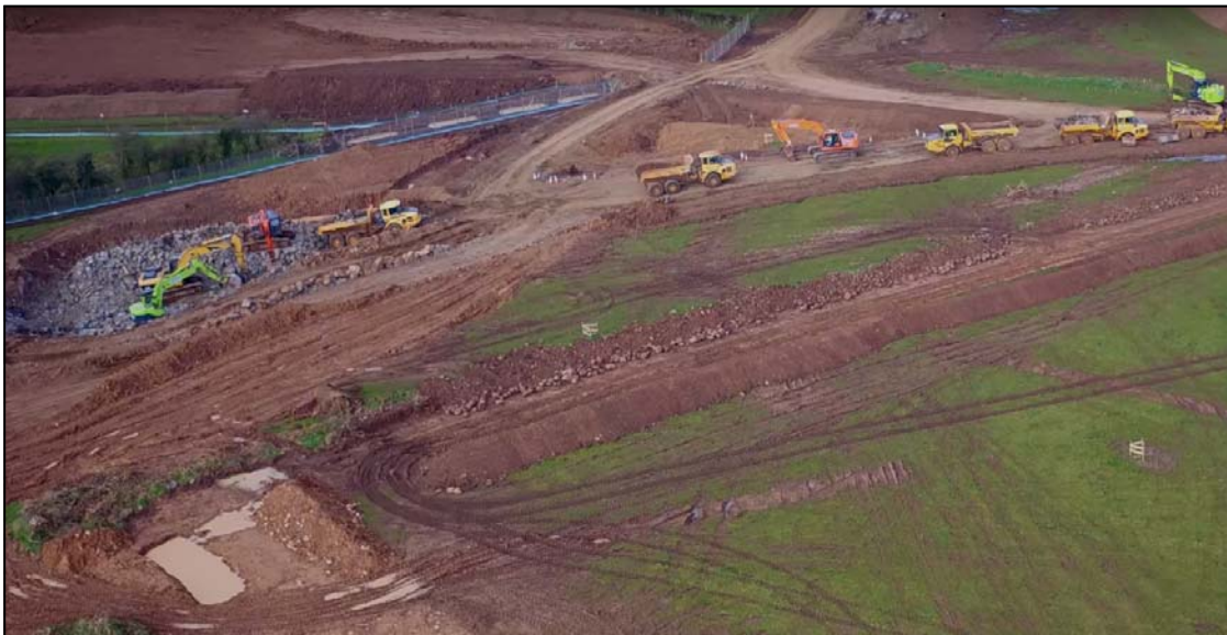
The Randalstown to Toome section of the A6 Dualling scheme at Aghnaloughan Road
