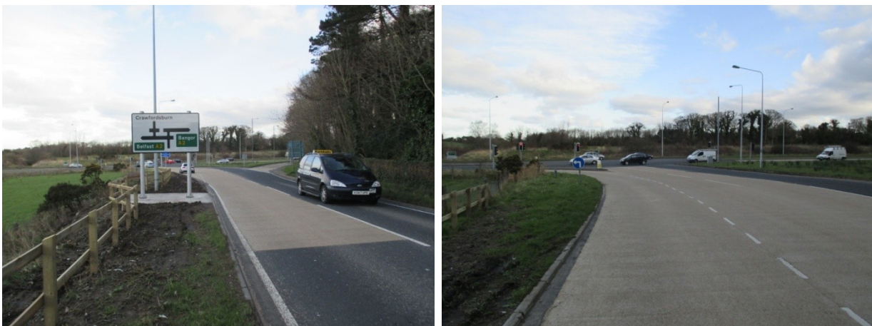
High friction surfacing on Ballysallagh Road on approach to A2 Belfast Road.
