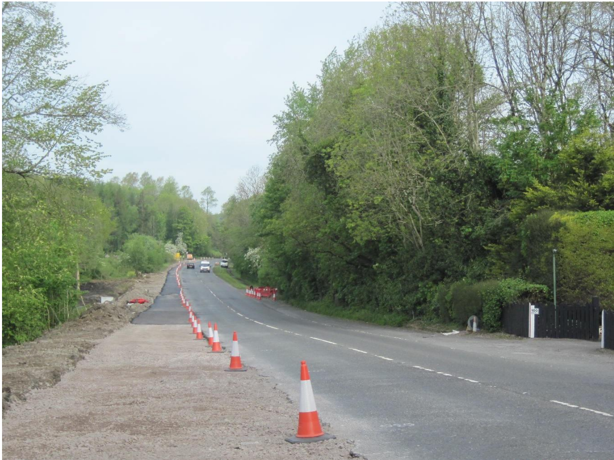
A4 Belfast Road at Dolan's Ring – commencement of right turning lane scheme
