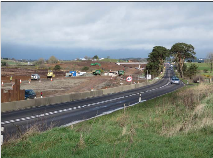
Earthworks activity adjacent to the Frosses trees on the A26 Dualling Scheme.
