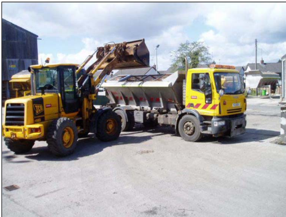
Salt loading one of the gritting lorries
