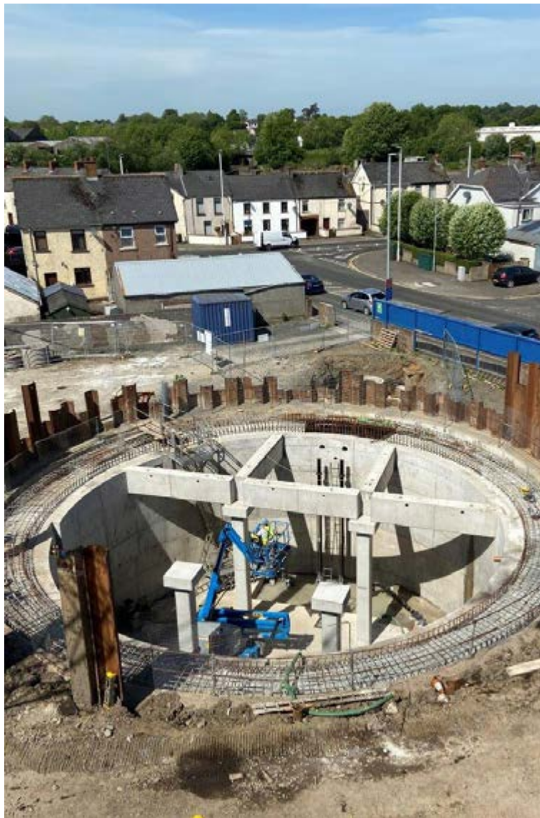
A look back to construction work on site at Wakehurst Road - June 2020
