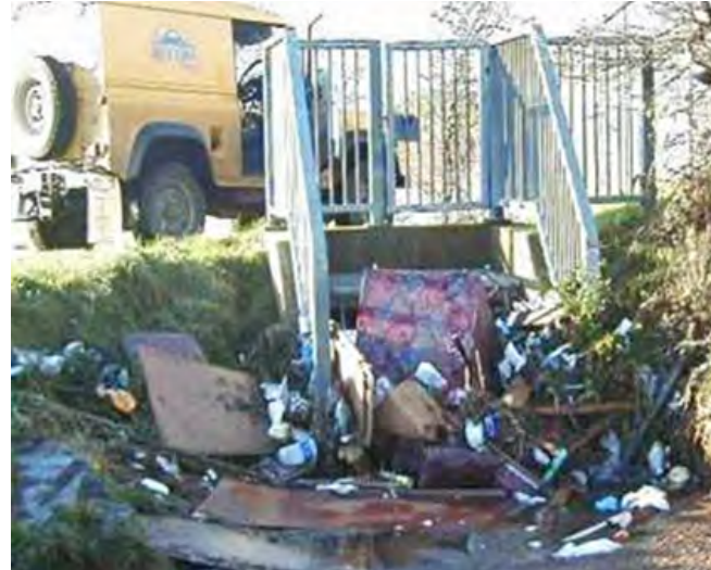
Grille blocked by debris washed down following heavy rain
