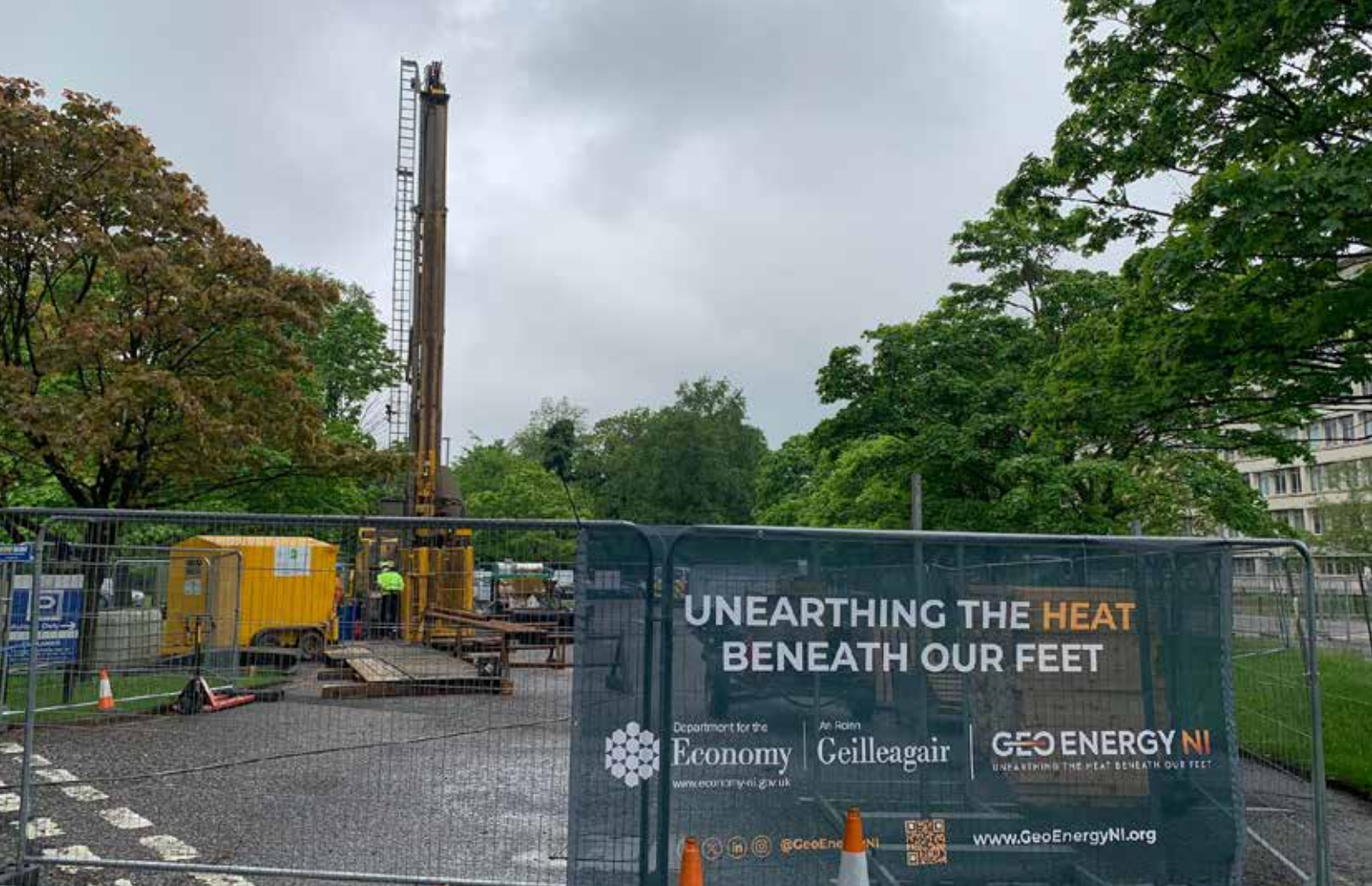
Drilling of a stratigraphic borehole outside Dundonald House on the Stormont Estate as part of GeoEnergy NI.
