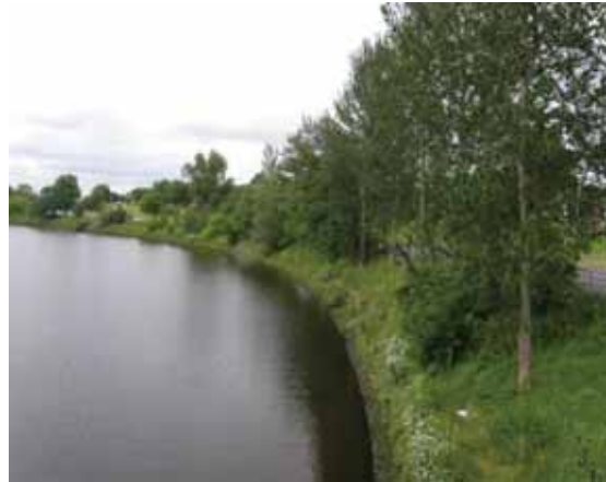
Plate 4.6 – View downstream along east bank of the Impoundment, from Kings Bridge showing hard engineered revetment at the base with a semi-natural grassland/tree & shrub mosaic along the top.
