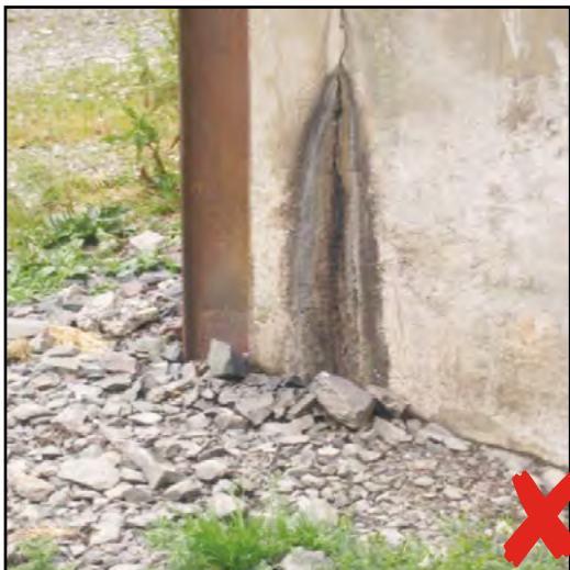
Photo 6 - Leaking silage clamp
