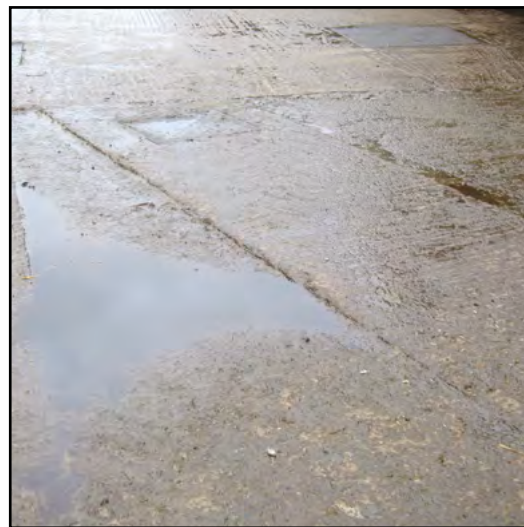
Photo 28 - Run-off from a frequently used roaming yard is slurry.
