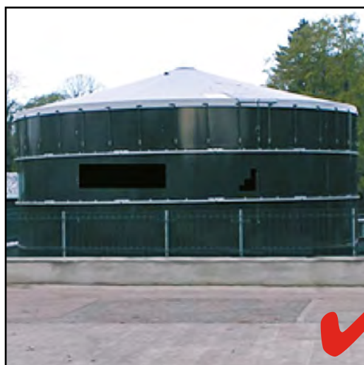
Photo 11 - Well maintained above ground slurry tank
