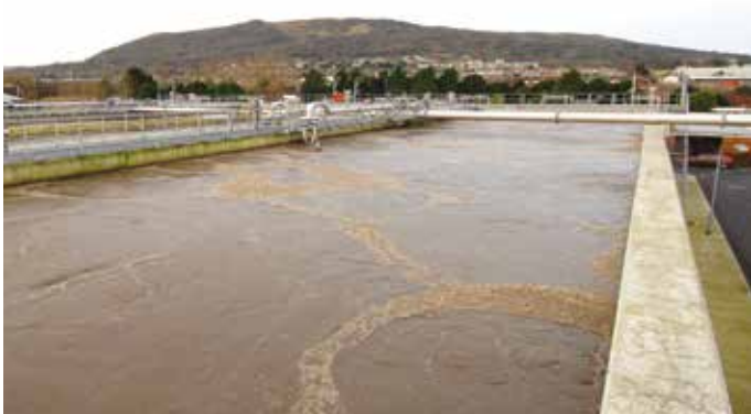
Figure 3.15 – Aeration Lanes at Whitehouse WwTW
