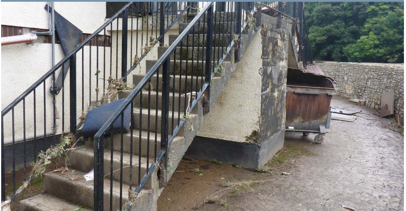
Figure 5.2-3: Flood wrack visible on railings of 'Three Mile House', within the Londonderry ASPFR with flood defence
