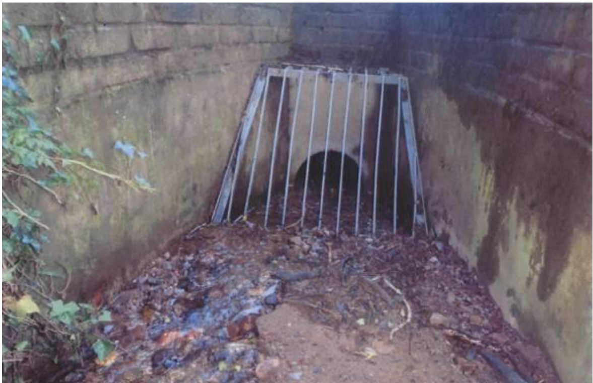
Photograph 7.5.6.1 - Ongoing problem with gravel accumulation at Ferndene Stream
