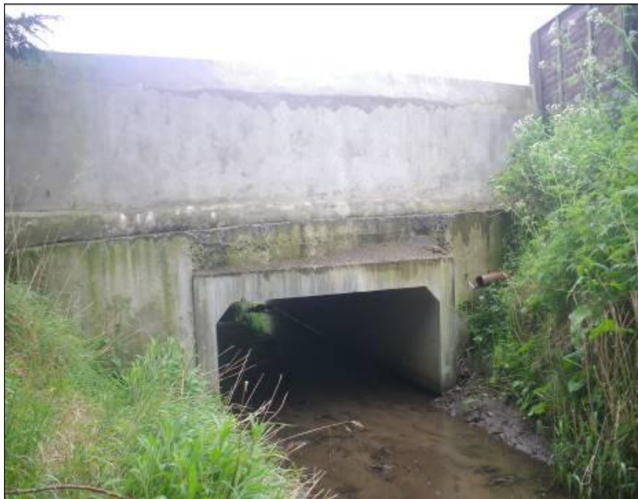
Photo 5.3.1.3 - Rivers Agency upgraded accommodation bridge on the Tirsogue Drain in Shanes Park, Lurgan
