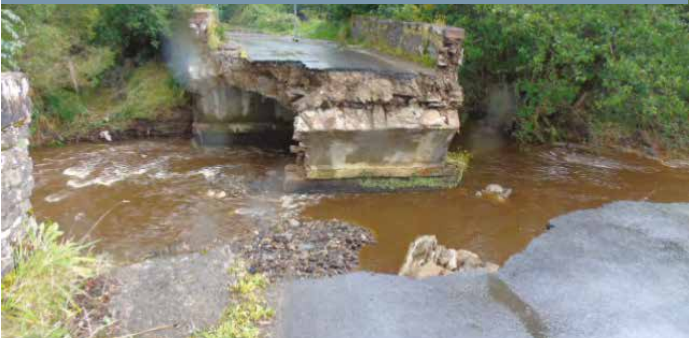
Figure 5.2-2: Collapse of the Glenrandal Bridge in Claudy (photo from NIFRA 2018) on the River Faughan, upstream of the Londonderry APSFR
