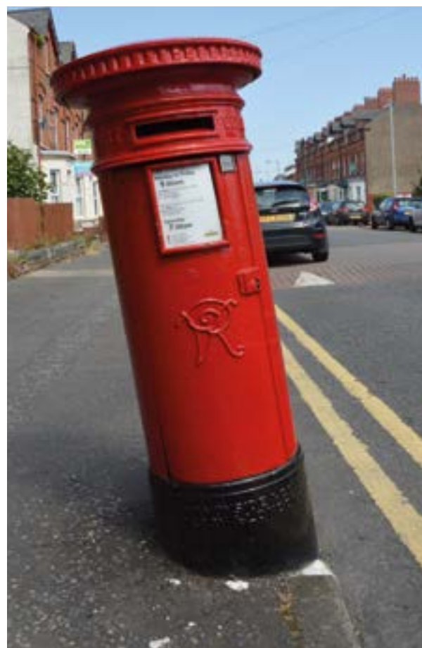
A Grade 'A' Listed Victorian Pillar Box on Agincourt Avenue, Belfast, damaged, probably by impact from a car
