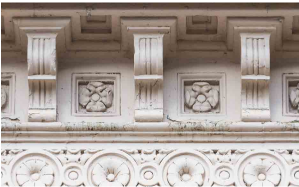
Plaster detail, Assembly Rooms, Belfast (Photo credit UAH David Bunting).
