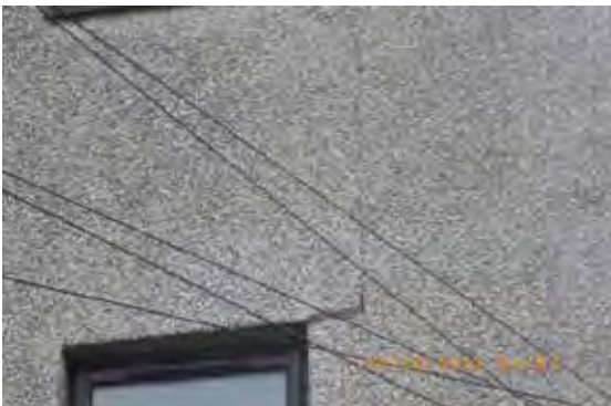
Figure 6.5 Crack running down the rear elevation
