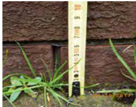
Figure 7.27 Non compliant DPC level (below 150mm)
