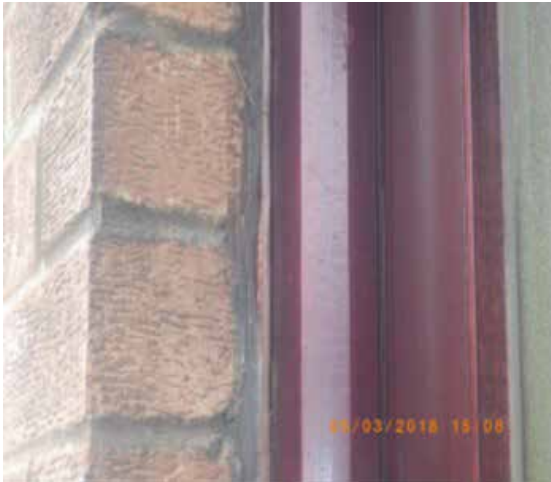
Figure 7.38 Defective perimeter seal (door)
