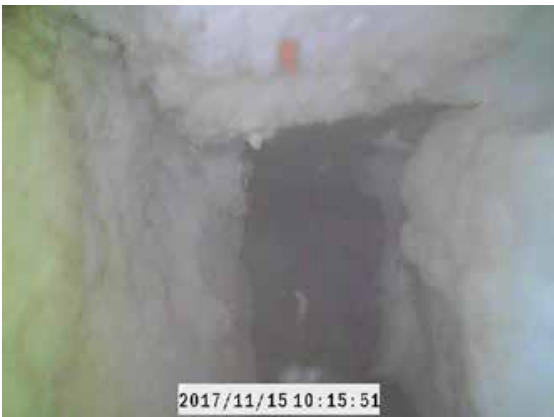
Figure 8.5 Voids in the foam CWI
