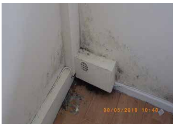
Figure 6.10 Damp on the internal wall
