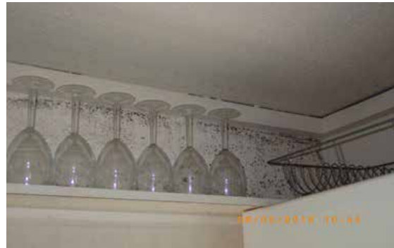
Figure 6.6 Condensation in the kitchen
