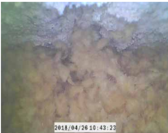
Figure 6.32 Void in the CWI
