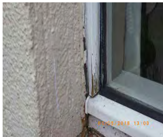
Figure 7.32 Defective perimeter seal (window)
