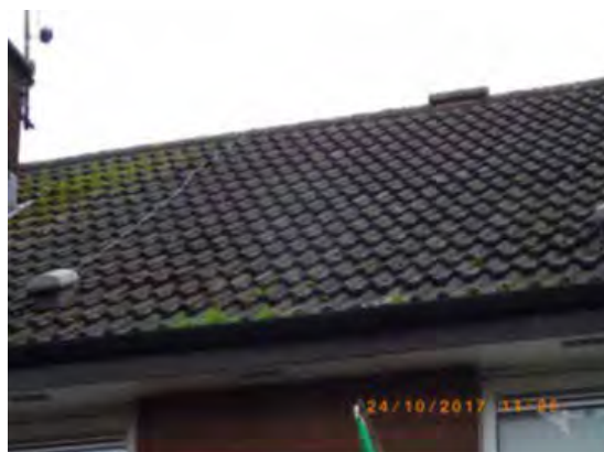
Figure 6.15 Vegetation growth in guttering (front) elevation.
