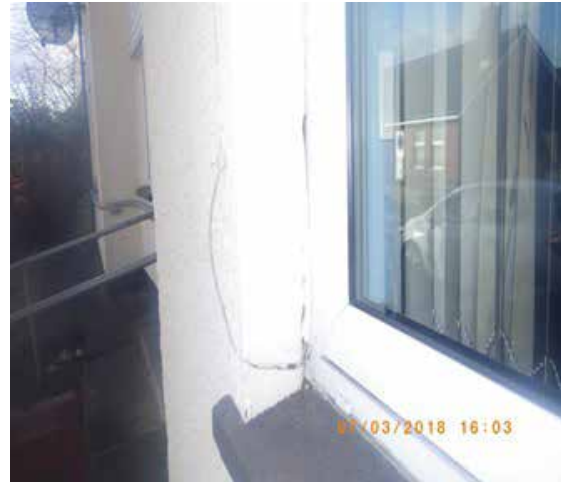
Figure 7.39 Defective perimeter seal (window)
