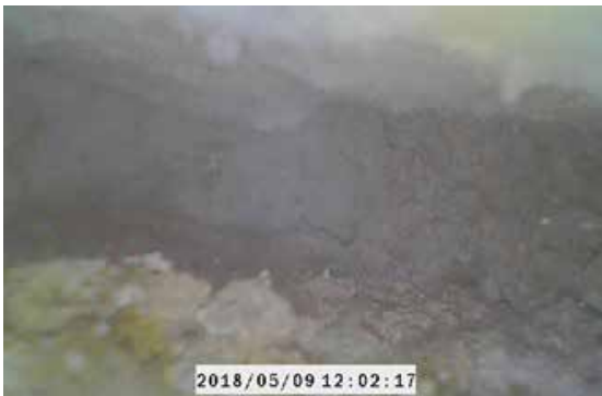
Figure 7.41 Void in the CWI installation
