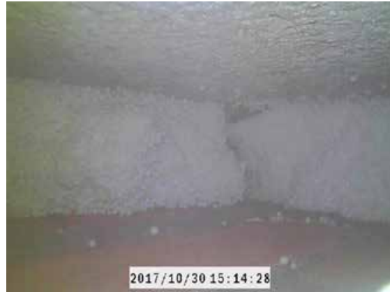
Figure 7.9 Void in the CWI installation
