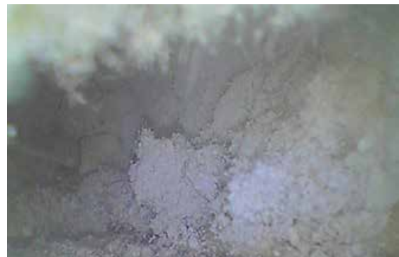
Figure 7.45 Void in the CWI installation
