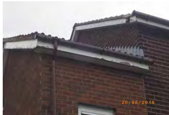
Figure 7.53 Damaged soffit and fascia
