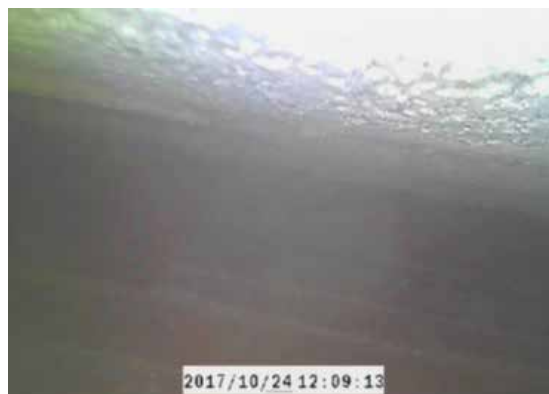
Figure 6.25 Void in CWI
