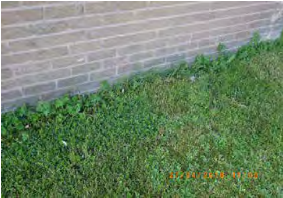
Figure 7.47 Non compliant DPC level (below 150mm)
