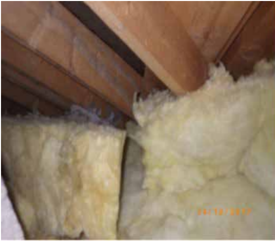
Figure 8.23 Eaves blocked with loft insulation
