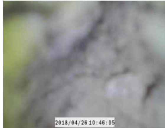
Figure 6.33 Inadequate CWI density
