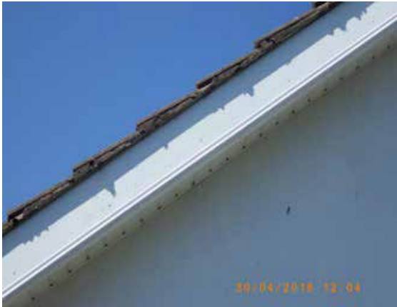
Figure 8.20 Damaged verge board
