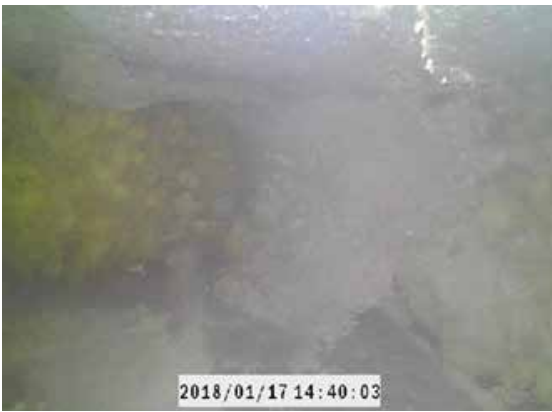
Figure 7.7 Void in the CWI installation and debris bridging the cavity
