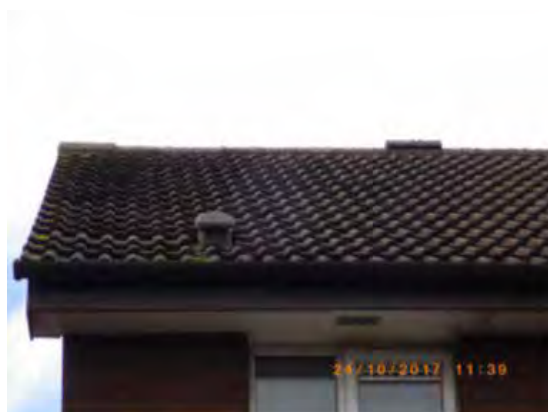
Figure 6.16 Vegetation growth in guttering (rear) elevation.
