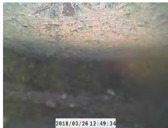
Figure 7.46 Void in the CWI installation
