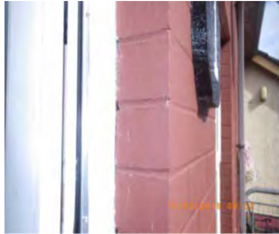
Figure 7.31 Defective perimeter seal (door)
