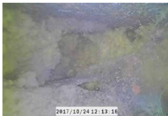
Figure 6.24 Void and debris in CWI
