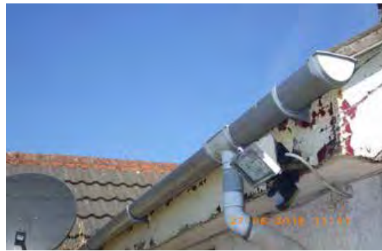
Figure 7.52 Damaged soffit and fascia
