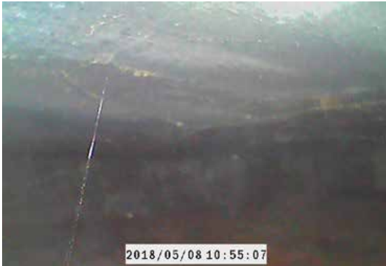
Figure 6.12 Voids and debris in the cavity
