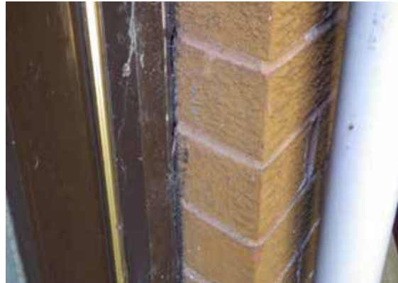
Figure 7.56 Defective perimeter seal (door)
