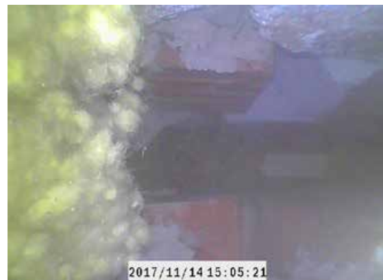
Figure 8.4 Voids and debris in the fibre CWI
