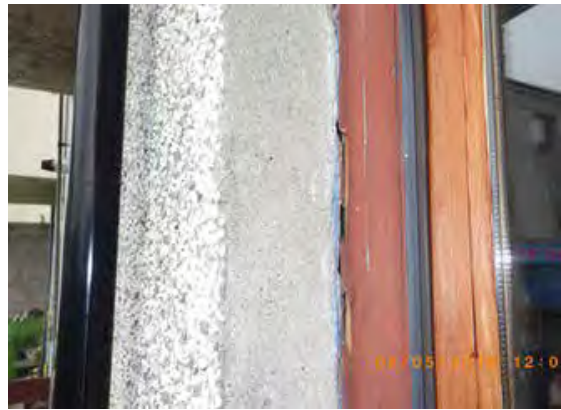
Figure 7.16 Defective perimeter seal between door and wall
