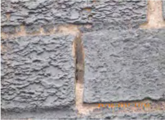
Figure 6.18 Mortar erosion (side) elevation
