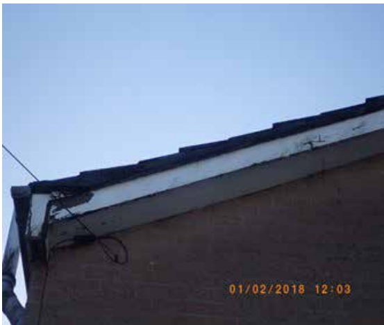
Figure 7.30 Compromised verge board
