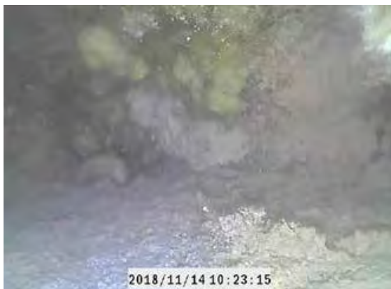
Figure 8.3 Voids and debris in the fibre CWI
