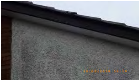
Figure 7.19 Damaged roof - Cracked verge mortar
