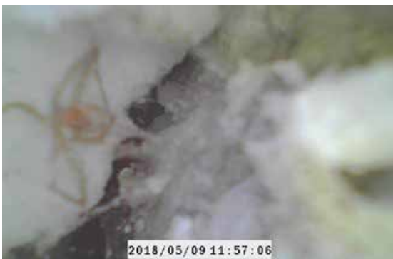
Figure 7.42 Void in the CWI installation
