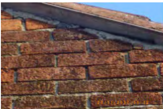
Figure 7.35 Compromised mortar joint
