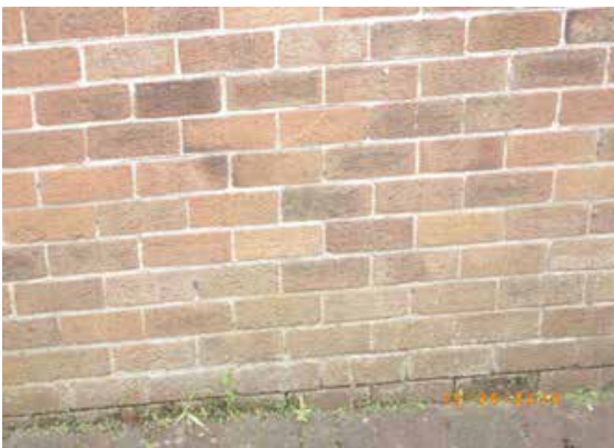
Figure 7.55 Non-compliant DPC level (below 150mm)
