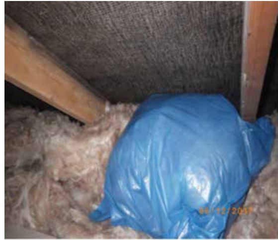
Figure 8.24 Eaves blocked with loft insulation
