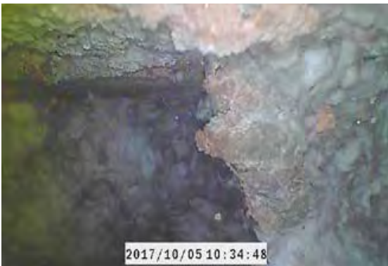
Figure 7.8 Void and debris bridging the cavity
