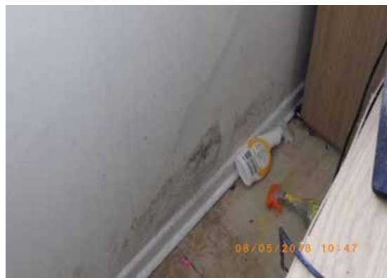
Figure 6.11 Damp on the bedroom wall
