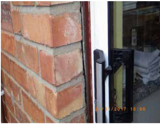
Figure 8.21 Defective perimeter seal (door)
