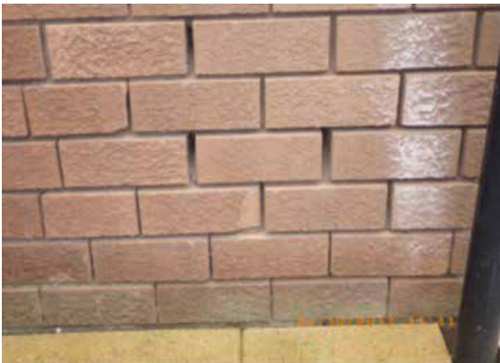
Figure 6.19 Mortar erosion (rear) elevation
