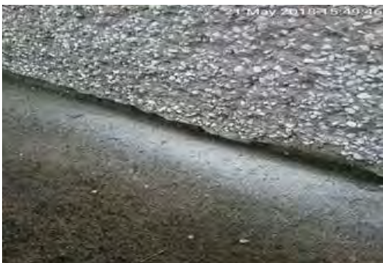
Figure 7.21 Non-compliant DPC level
