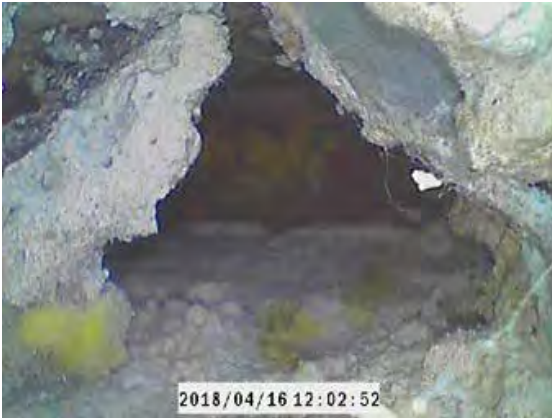
Figure 7.6 Void in the CWI installation
