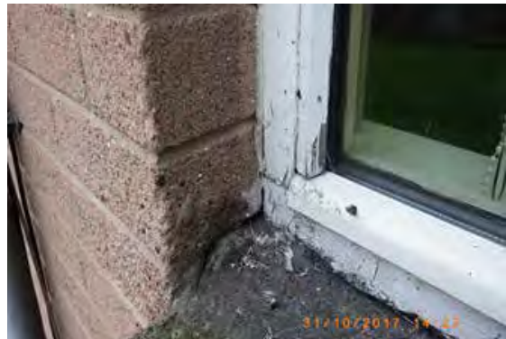
Figure 7.17 Defective perimeter seal between window and wall
