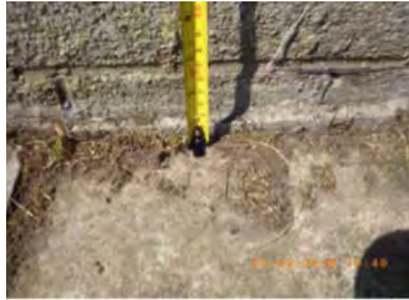
Figure 8.14 Non-compliant DPC level (below 150mm)
