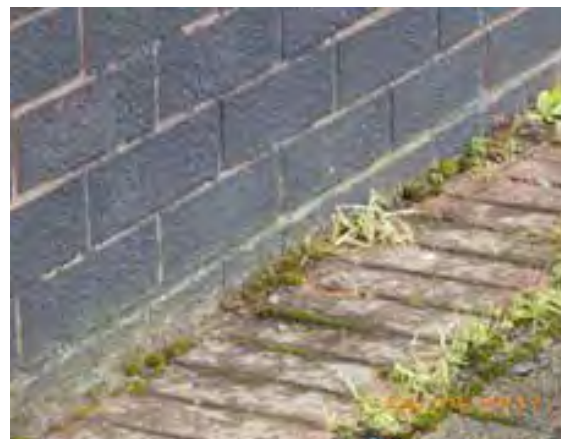
Figure 7.28 Non compliant DPC (below ground level)
