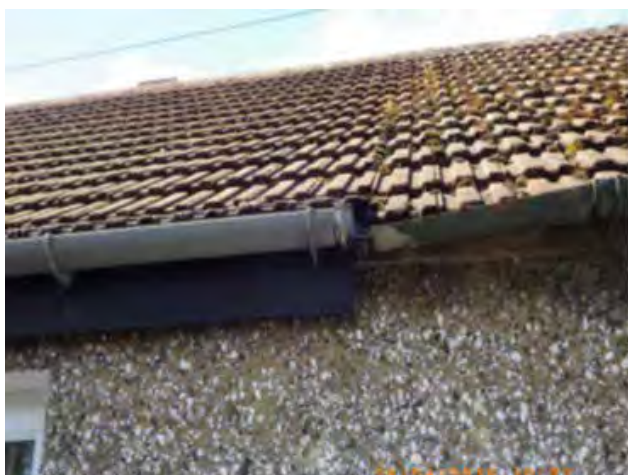
Figure 6.28 Broken guttering joint
