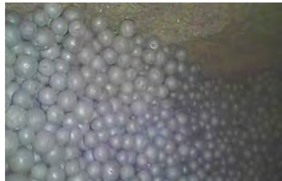
Figure 7.44 Void in the CWI installation
