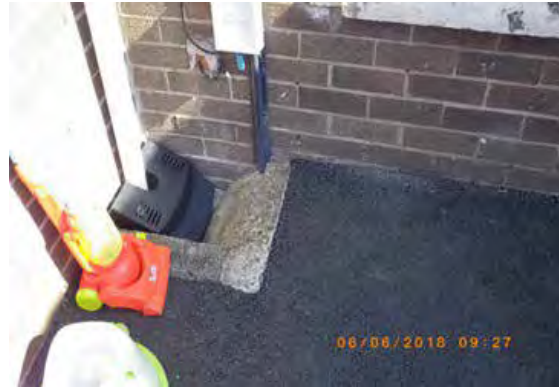
Figure 7.48 Non compliant DPC level (below the Tarmac)
