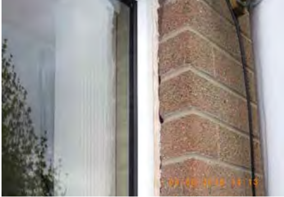
Figure 8.22 Defective perimeter seal (window)
