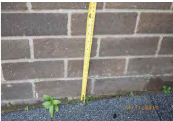
Figure 8.13 Non-compliant DPC level (below 150mm)
