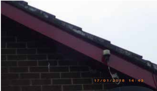
Figure 7.18 Damaged roof – Cracked verge mortar
