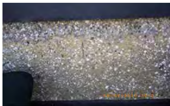
Figure 6.30 Crack in the render
