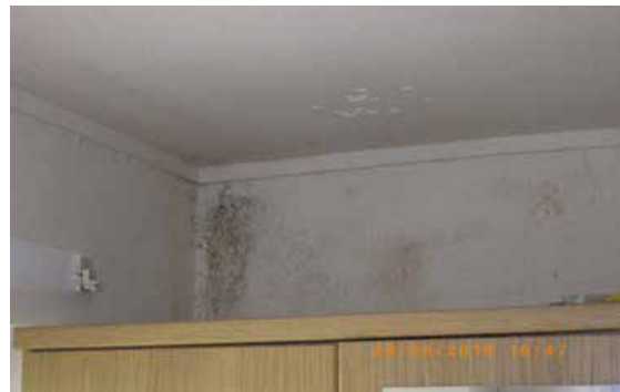
Figure 6.7 Condensation in the bedroom
