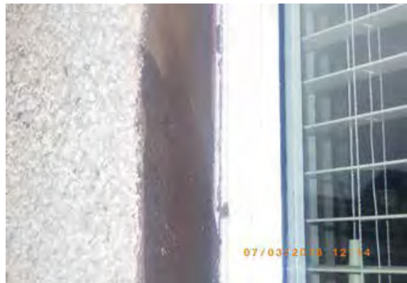
Figure 7.57 Defective perimeter seal (window)
