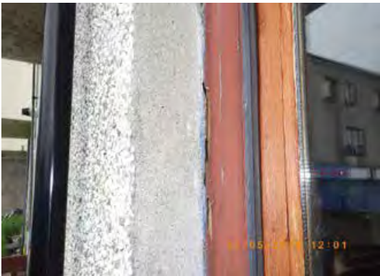
Figure 6.4 Compromised perimeter seal (door)
