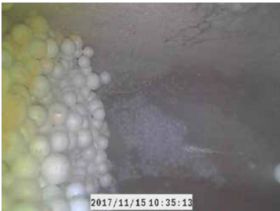
Figure 8.8 Voids and debris in the bead CWI
