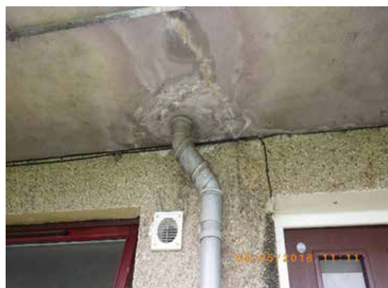
Figure 6.2 Water damaged roof
