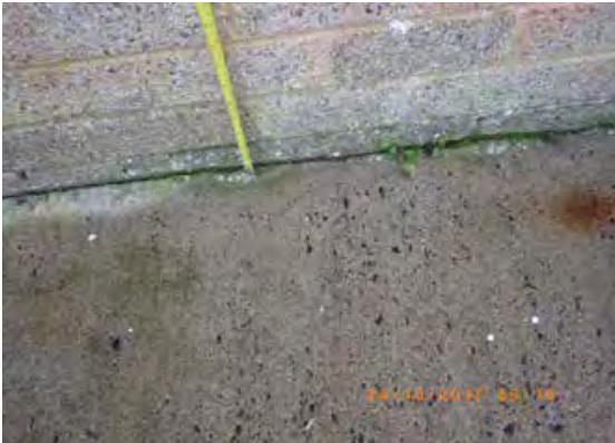
Figure 7.54 Non-compliant DPC level (below 150mm)
