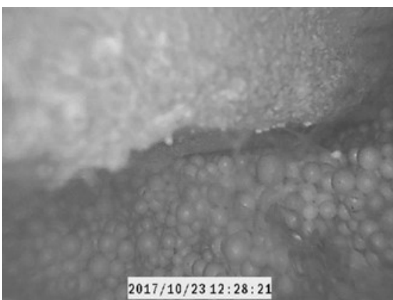
Figure 7.43 Void in the CWI installation
