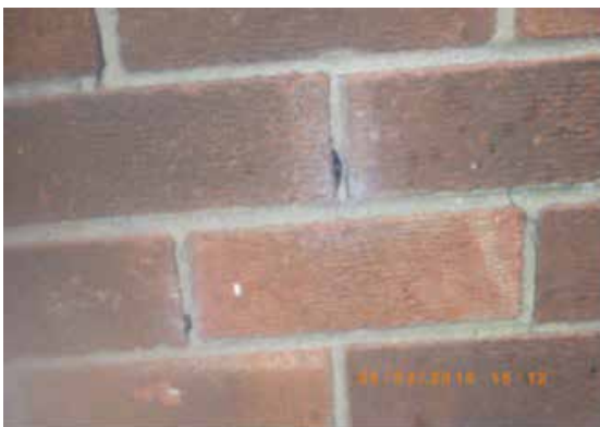
Figure 7.34 Compromised mortar joint
