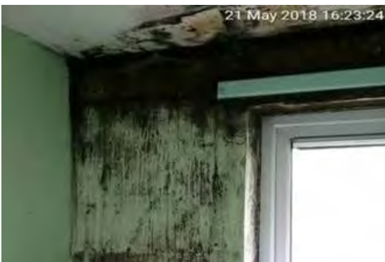
Figure 7.14 Damp and condensation
