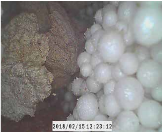
Figure 7.23 Debris in cavity and void in CWI
