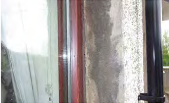
Figure 6.3 Compromised perimeter seal (window)
