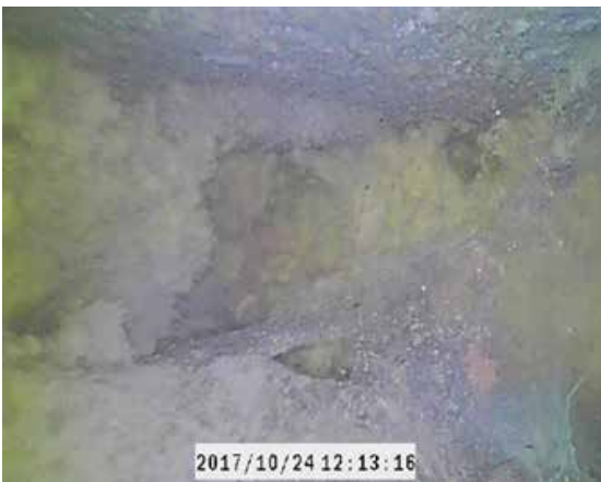
Figure 7.24 Debris in cavity and void in CWI
