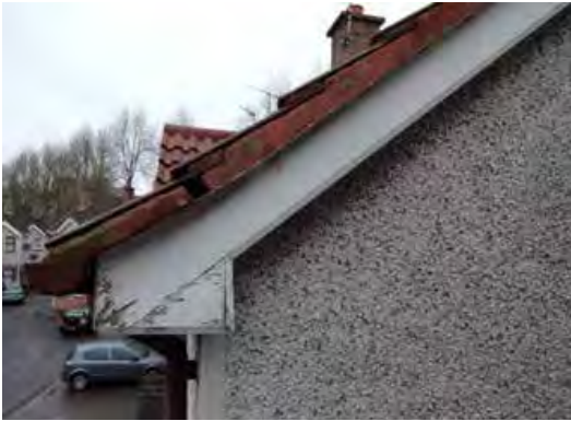
Figure 8.19 Damaged verge board
