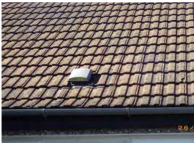
Figure 6.27 Broken roof tile
