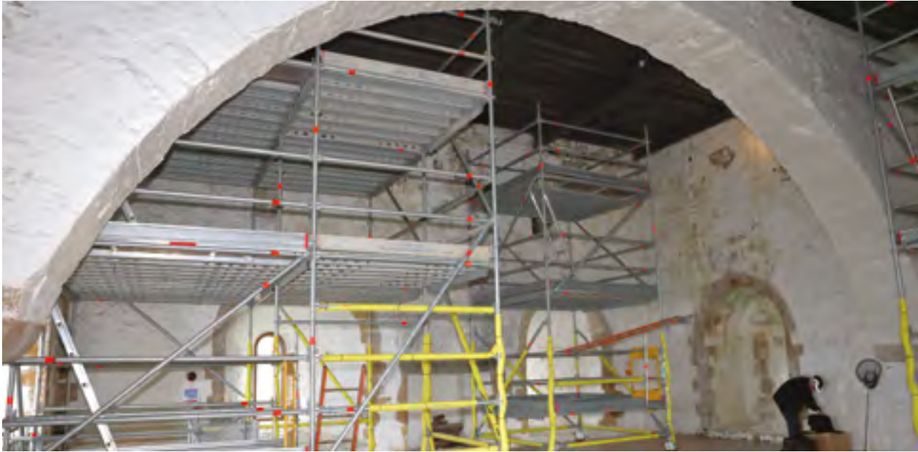
Conservation work in progress on the upper floor of the keep, Carrickfergus Castle, Co. Antrim, photo: HED
