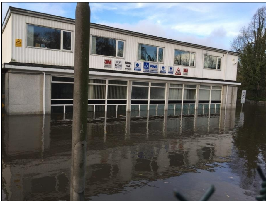
Figure 5.7 Flooding at PWS, Greenbank Industrial Estate
