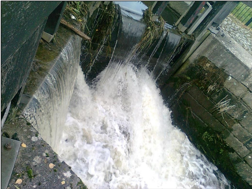
Figure 5.2 Overtopping of Lock Gates at Lock No.3 (October 2011)
