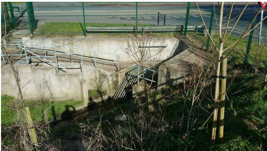
Figures 5.20 & 5.21 – Existing watercourse and culvert adjacent to A3 Portadown Road at Linsey’s Heights / Linsey’s Hill
