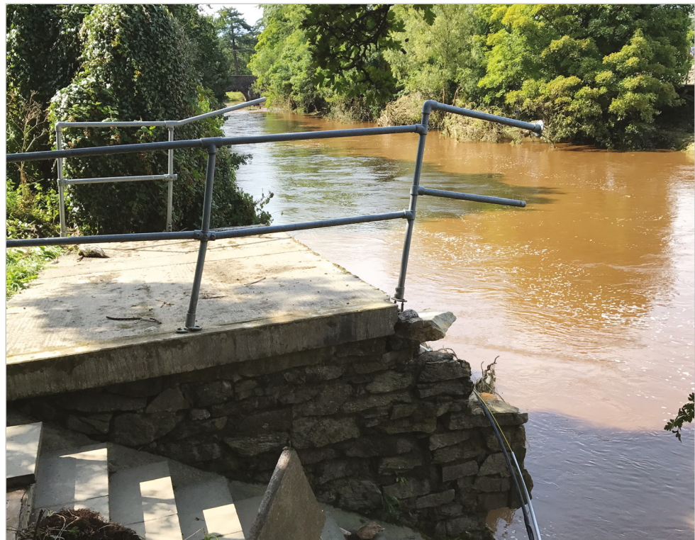
Drumahoe gauging station on River Faughan washed away by flood waters.
