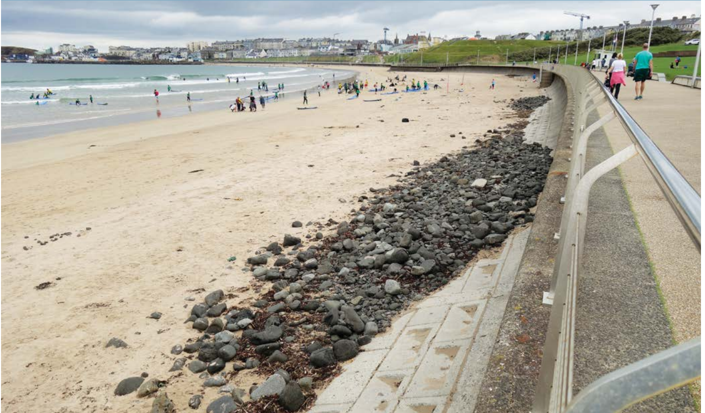
Photograph 4. Sea wall that resulted in lowering of the beach at West Strand, Portrush
