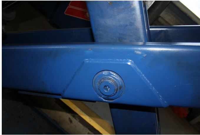
Typical outer box section – outside face with remedial steel plate
